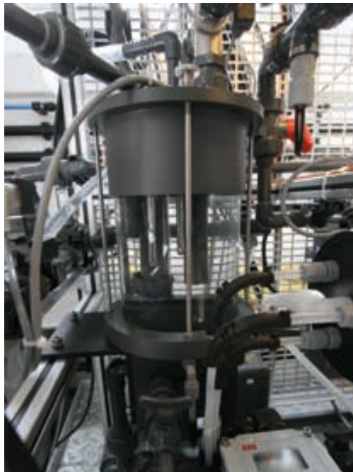
A Ferry Box system, installed onboard MV Armorique (Brittany Ferries). (© Yann Fontana / Station Biologique de Roscoff)
